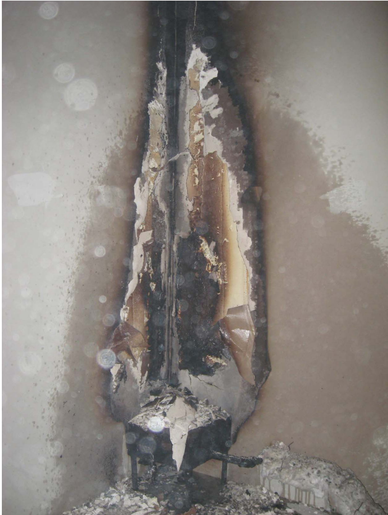
Post-test damage beneath gypsum wall.
